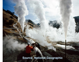
Source: National Geographic U.S.'s first geothermal power plant, Mayacama Mountains, California, turned 50 in 2009
